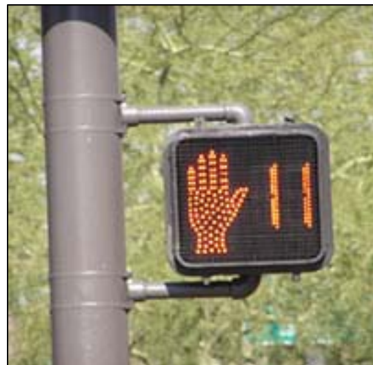
Countdown pedestrian signal heads help make safer pedestrian crossings (Source: www. http://guide.saferoutesinfo.org )
